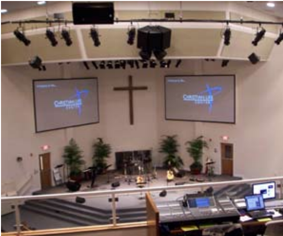
An extensive AV system designed by Thorburn Associates enhances New London Church.
